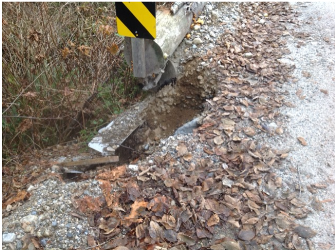
right bank upstream erosion
